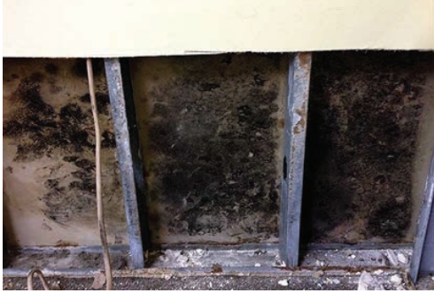
Mold and rust caused by uncontrolled moisture
