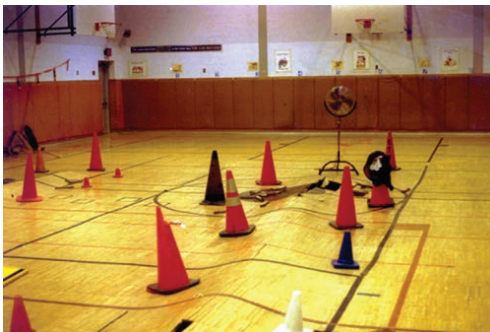
Damage from rain water entering at the roof-wall connection and draining inside the wall, to the under-floor slab
